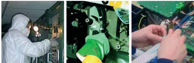
above: left: high pressure cleaning of contaminated control cabinet middle: cleaning contaminated control cabinet, right: documentation on printed circuit board.
